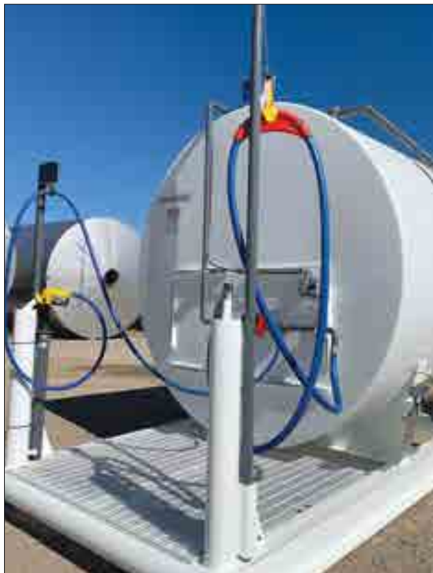
Fig 18 - Pump and Delivery system
