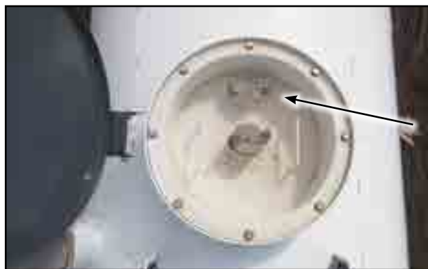
Fig 22 - Inside Spill Box is the Dip Port
