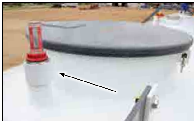
Fig 9 - Containment Inspection Port w/ Leak Detection Gauge
