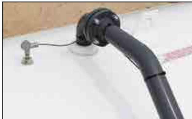
Fig 16 - MECO Overfill Alarm is connected to the fill tube
