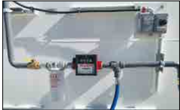
Fig 24 - Pump filter and meter
