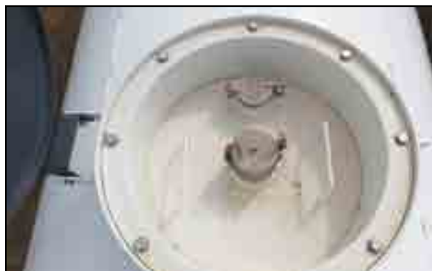
Fig 19 - Inside the Spill Box on standard tank
